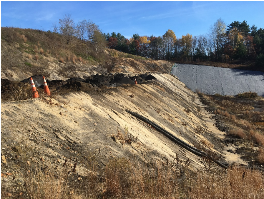
Photo 2: Landfill working face with flatter benched slope constructed. The photograph was taken from near the west side of the active area and looking east.
