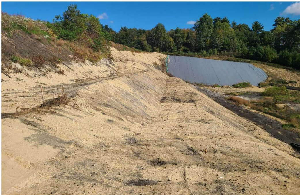
Photo 2: Active cell of the landfill with reduced steep slope at working face looking east from east side of active cell.
