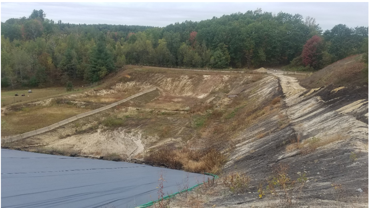
Photo 2: Active cell of the landfill with steep slope at working face looking west.
