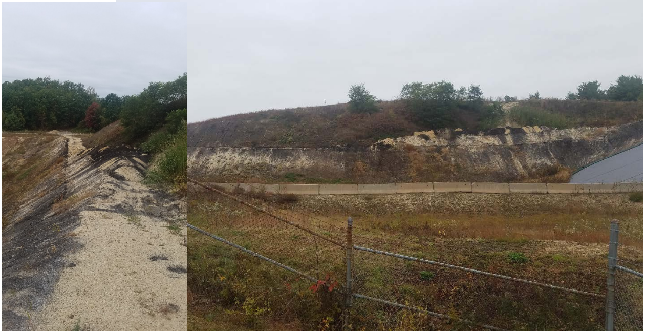
Photo 1: Active cell of the landfill with steep slope at working face looking north (right photo) from leachate collection building and east from east side of active cell (left photo)
