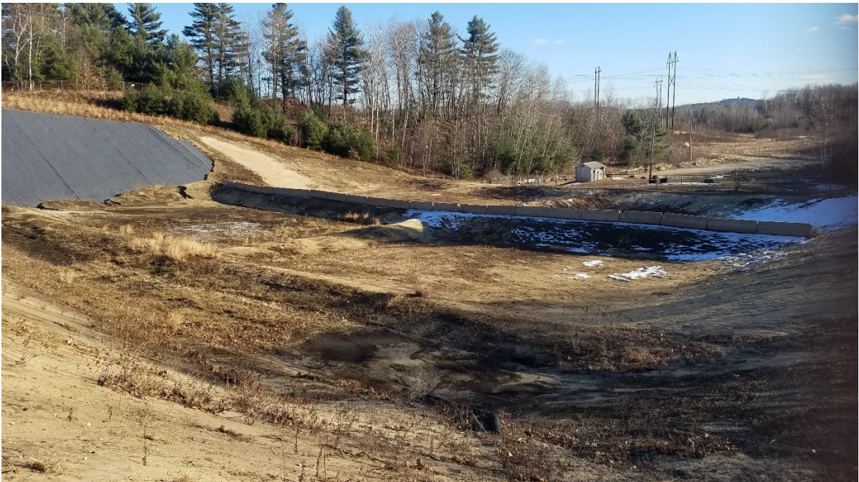
Photo 4: Landfill cells not currently in use looking southeast from east side of active cell.
