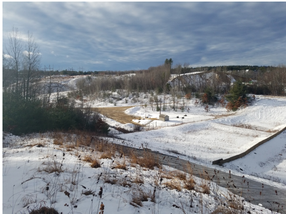
Photo 2: Limited woody vegetation growing near anchor trench.
