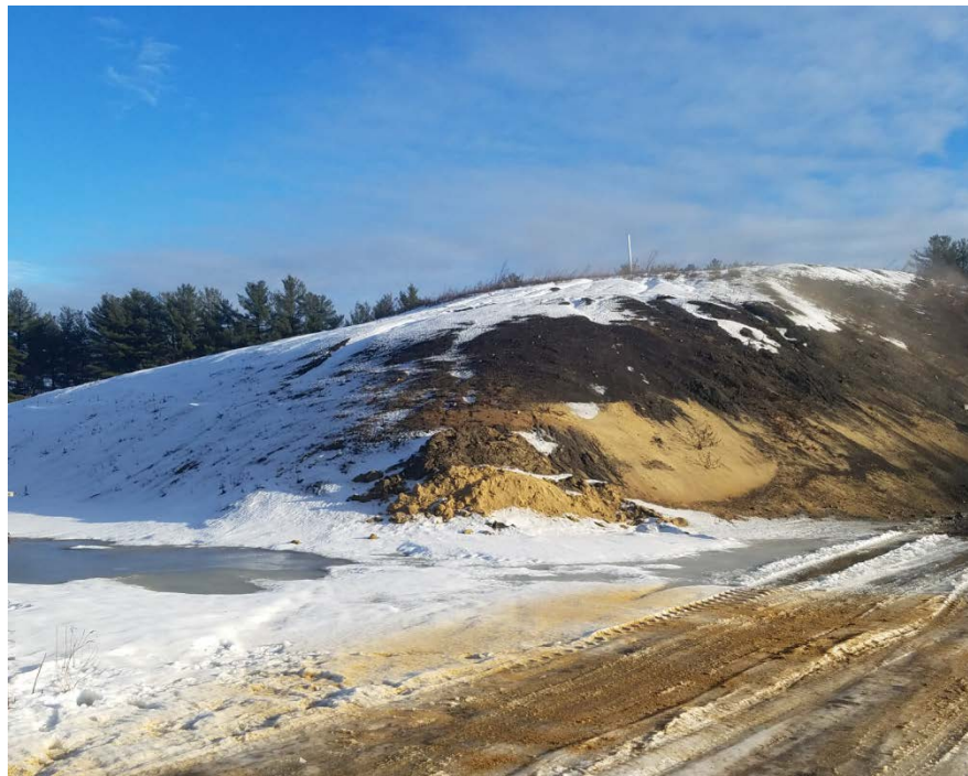
Photo 4: Area where limited erosion near active face of the landfill was repaired in 2016.
