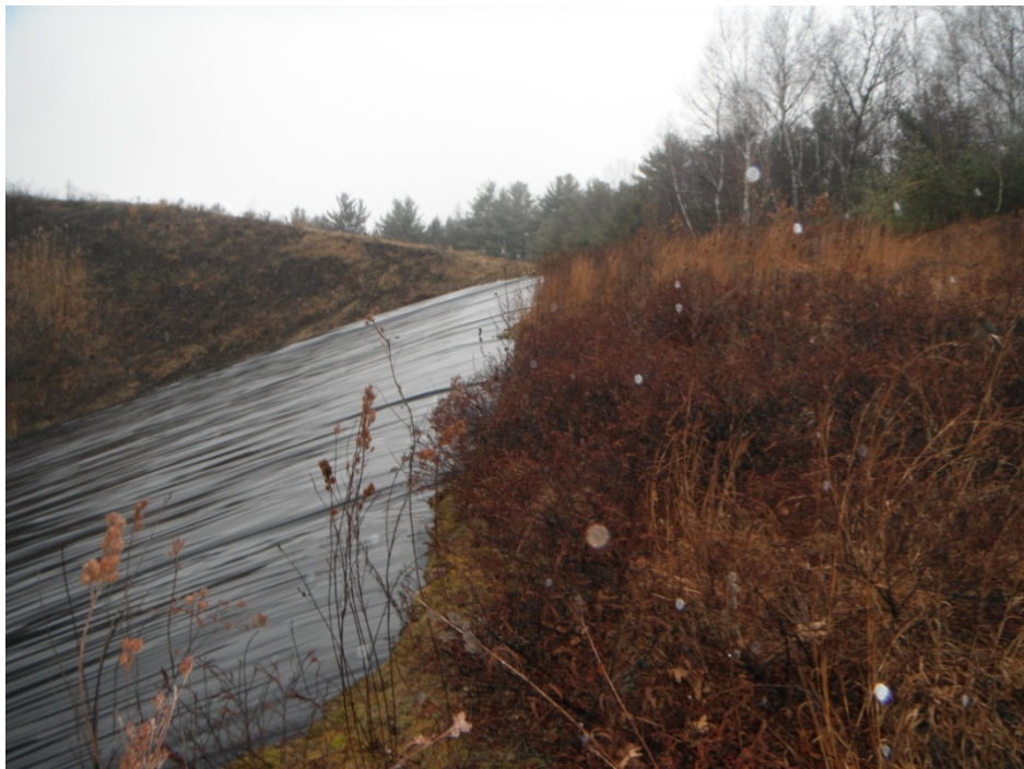
Photo 2: Limited woody vegetation growing near anchor trench.
